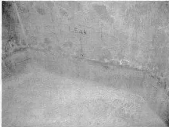
Figure 22: Water staining at cold joint in precast panel
