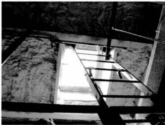
Figure 2: Radar access hatch
