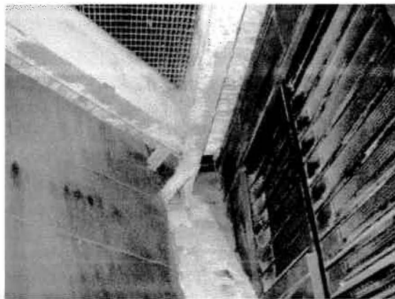
Figure 14: Water staining on sloped metal panels and structural steel at air intake plenum
