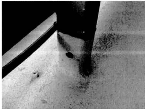
Figure 12: Hole in post railing
