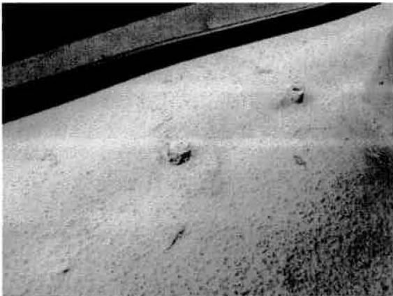
Figure 11: Discontinuity of deck traffic coating
