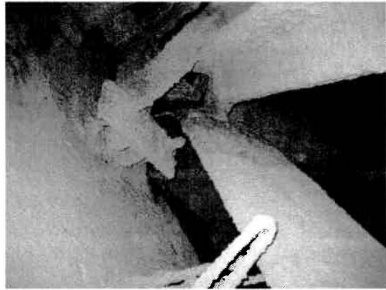
Figure 16: Staining noted in interstitial space at 45 degree bend in precast
